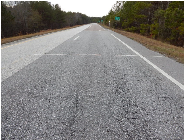
Figure 3. Top-Down Cracking of a Test Section on the NCAT Test Track.
