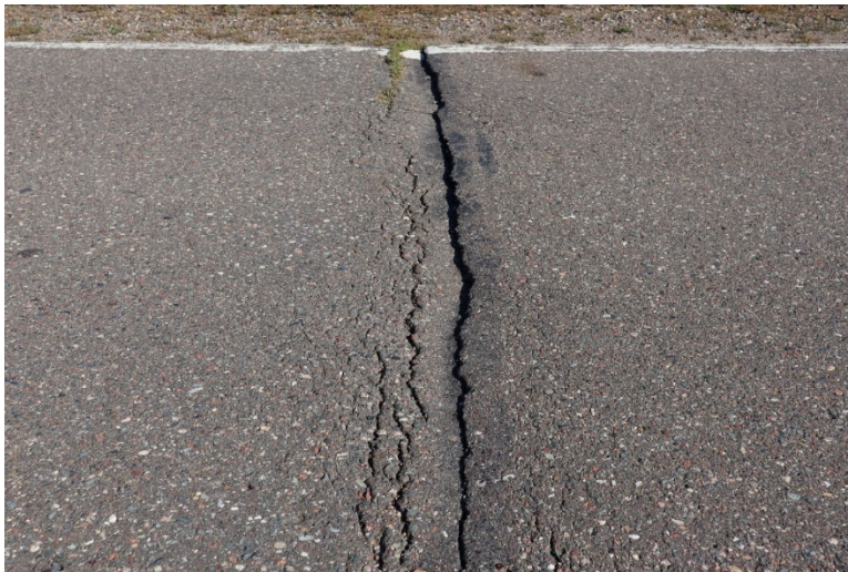
Figure 5. Thermal Crack in an Asphalt Pavement.
