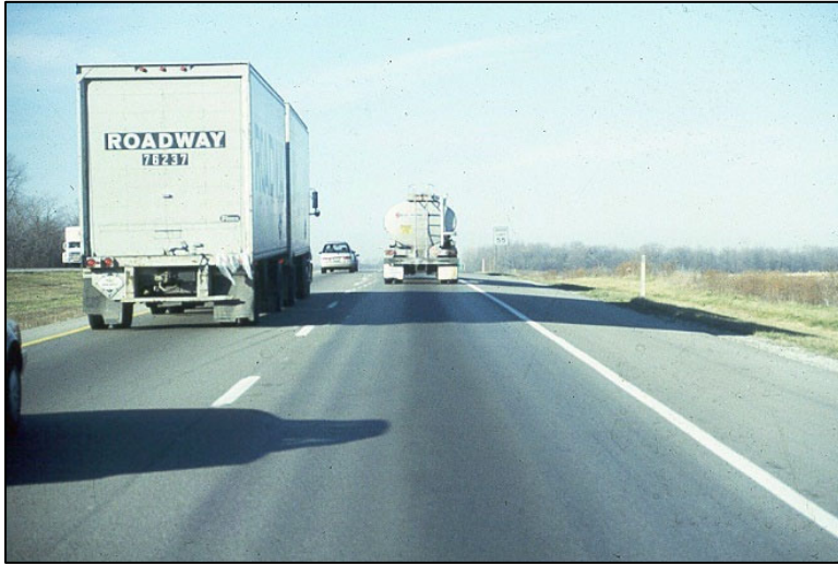
Figure 2. Rutting on an Interstate Pavement.
