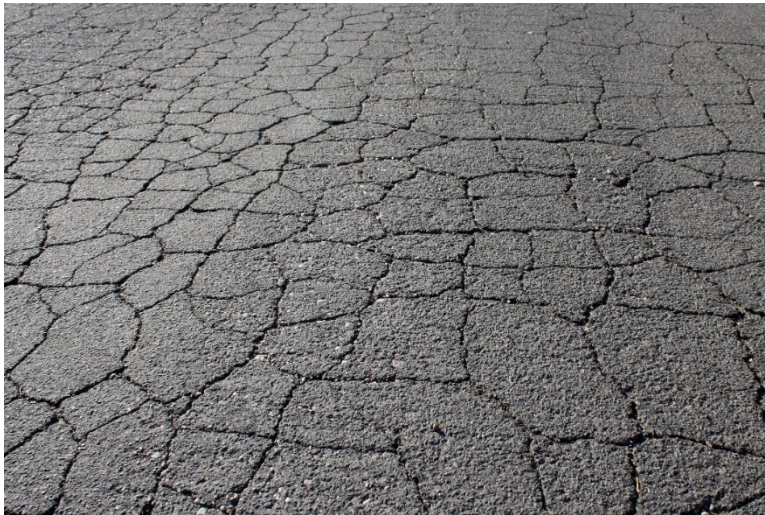
Figure 4. Extensive Fatigue Cracking of an Asphalt Pavement.
